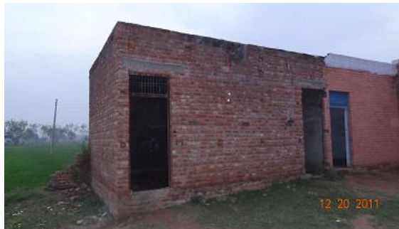
Construction of room for Govt. primary school, Village: Kotli Jawahar , Block: Bamial
