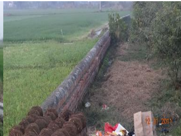
Construction of retaining wall of pond, Village Chaniewal, Block Dera Baba Nanak
