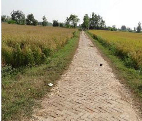
Construction of 4 ways of village deras Village: Rauwal Block: Dera Baba Nanak
